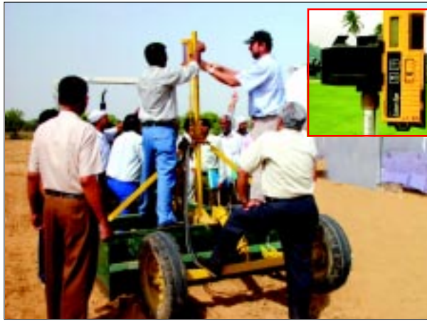
Fig. 11. Laser receiver being adjusted on the mast. Inset picture shows a close-up of a laser receiver.
