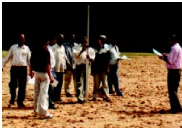
Fig. 17. Taking survey readings in the field with reference to a fixed datum.
